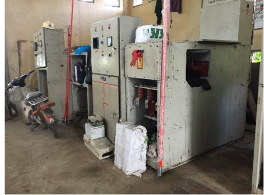
Shwe Pauk Kan Substation
