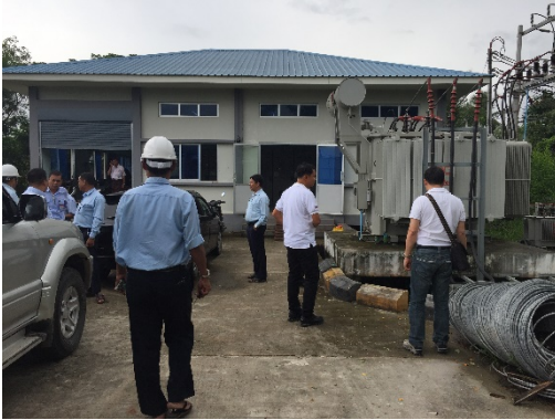
Wai Bar Gi Substation
