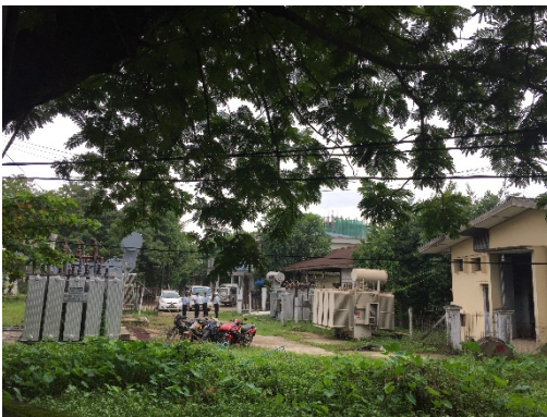
North Okkalapa Substation
