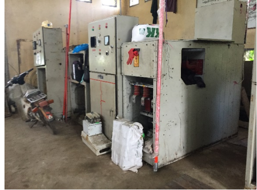
Shwe Pauk Kan Substation
