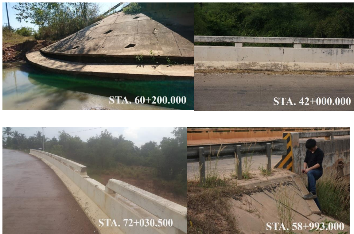
Figure 5.6-1 Damage of Bridge Slope Protection and Bridge Railings
