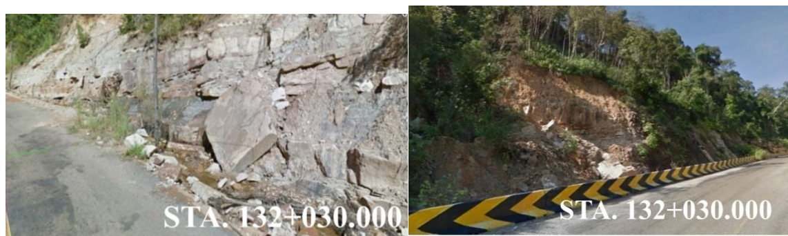
Figure 5.10-1 Rockfalls from Hillsides
